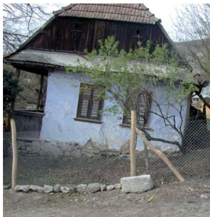
Tilting of building due to landslide movement
